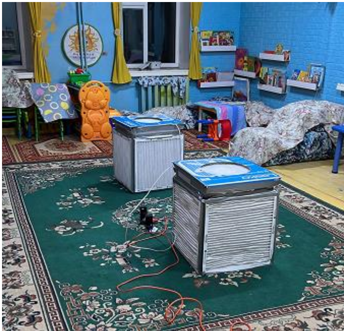
Figure B.4 C-R box filtration system in KG45
