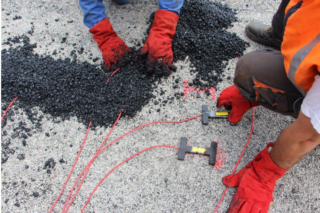
Figure 6.19: The H-gage sensors being placed for installation before being covered by virgin aggregate and petroleum bitumen asphalt pavement.
