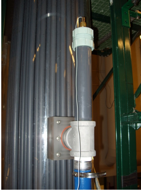
Fig. 5.4 – Conductivity probe (#2) inside a PVC tube at the liquid outlet
