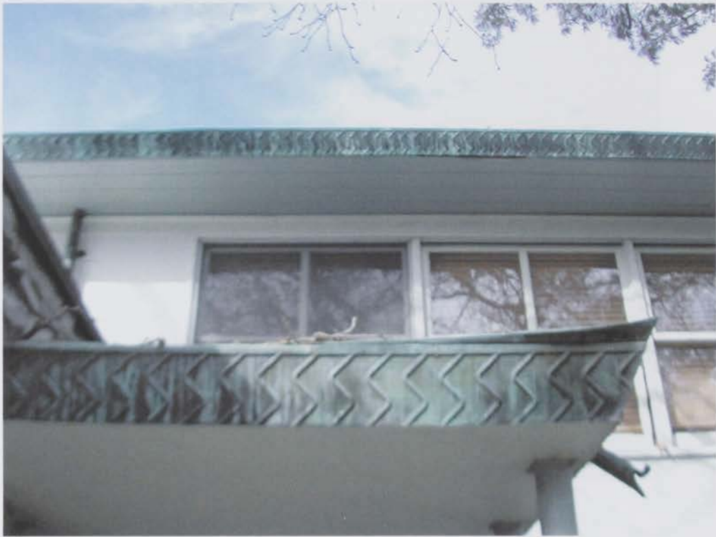
Fig. 39. Harris Armstrong House, flared copper gutter detail,
