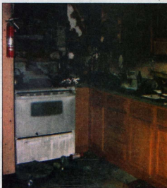
A grease fire started on the stove of Millbrook RCD Ozie Goodwin's apartment on Saturday. Goodwin's apartment suffered significant damage and other Millbrook residents have been temporarily displaced.
