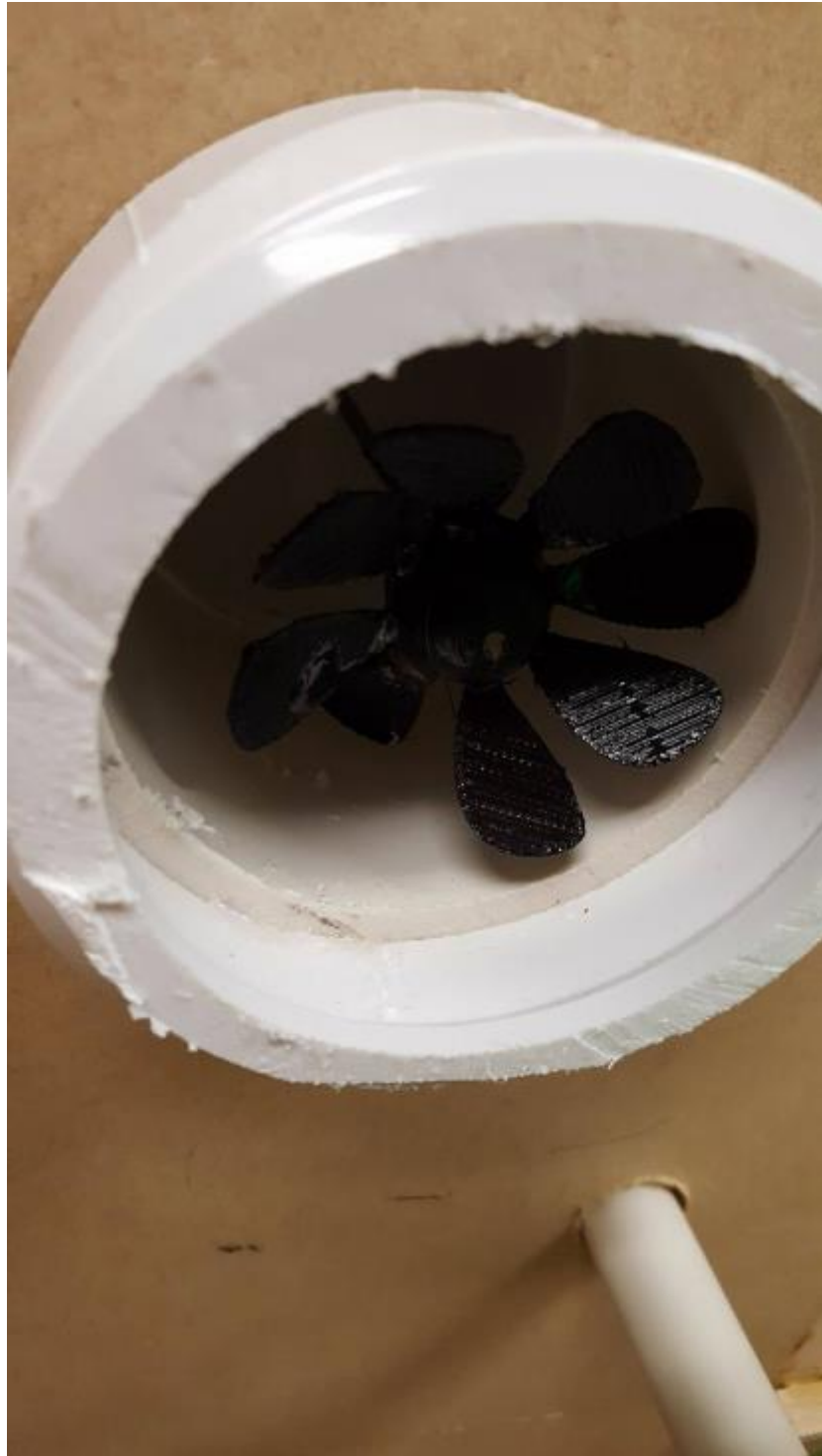
Figure 27: Picture of the fan inside the reservoir.
