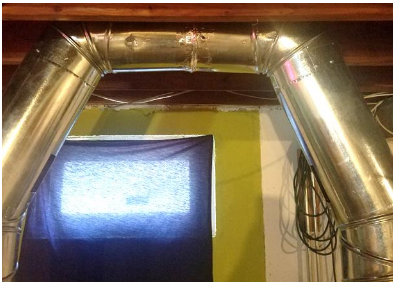
Figure 26: The supply duct vents are capped and meet at the apex of the archway.
