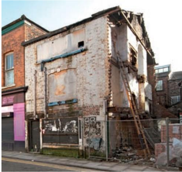
Figure 3: Three story workshop dwelling which is recognizable by a wide window facing the street, located on 88 Street in the Northern Quarter. (Taylor and Holder, 2008, page 13).
